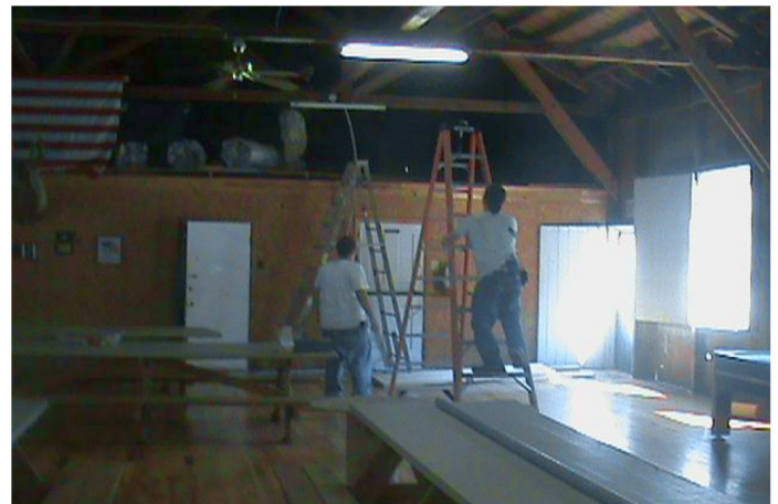
Lodge members working on installing the new electrical feed in the Dining Hall
